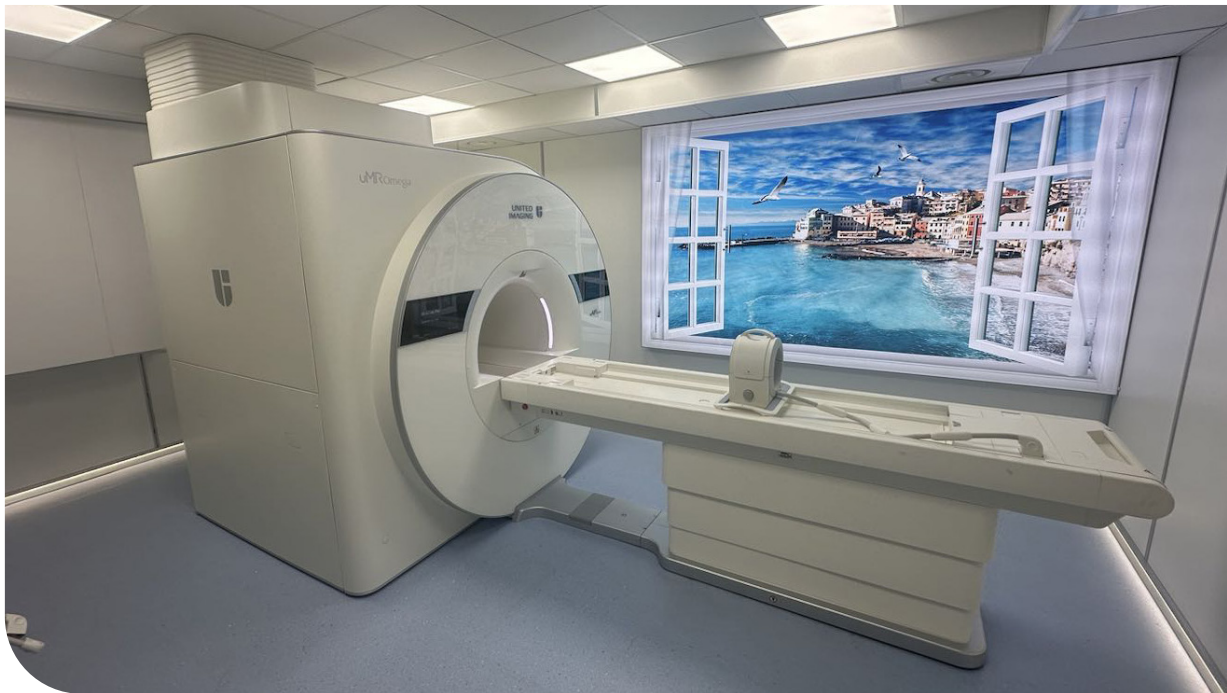
uMR Omega™ installed in Cobellis Clinic, Campania, Italy
